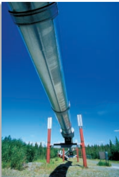
FIGURE 10 The Alaskan pipeline is cathodically protected by a parallel zinc cable.
